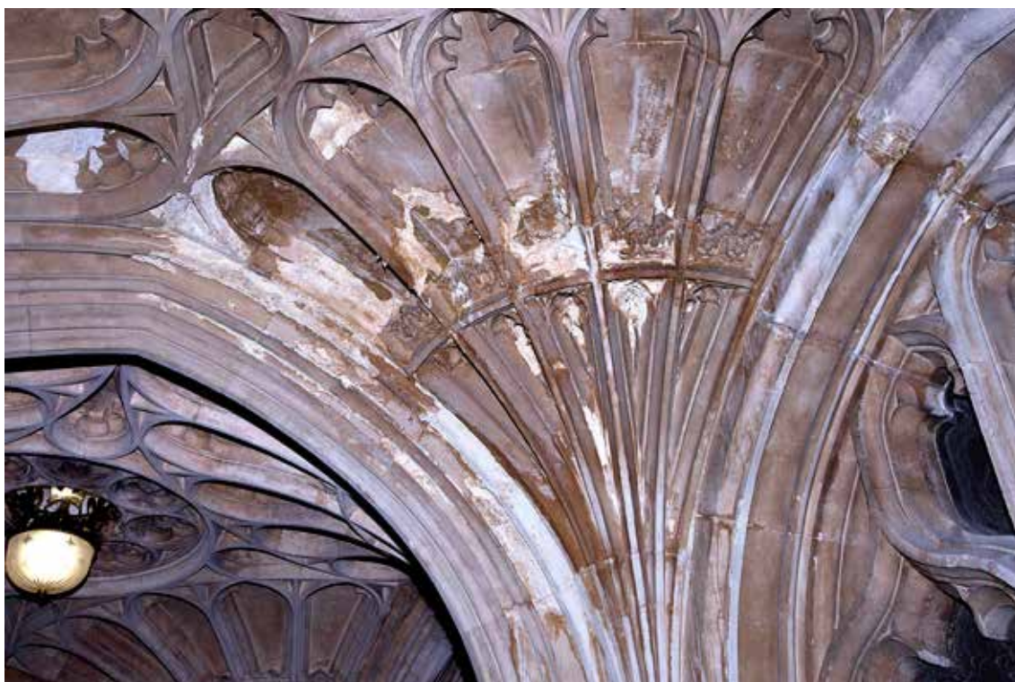
Figure 4: Water damage caused by a blocked roof gully
