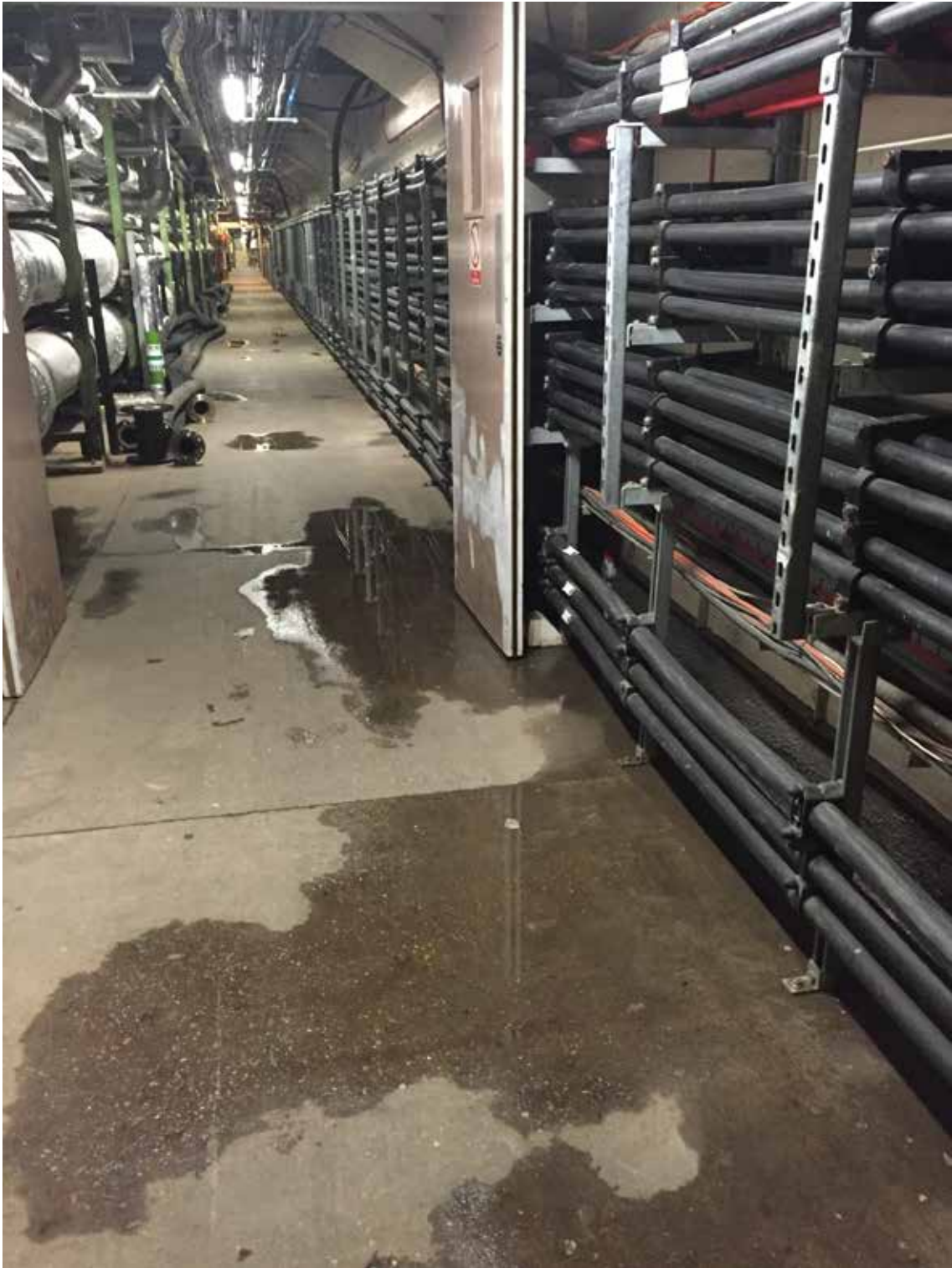
Figure 3: Water leaks in the basement
